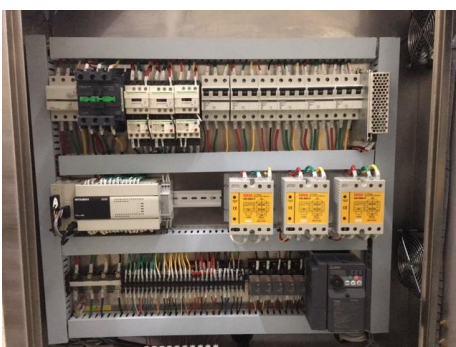
Control Box Mitsubishi, Schneider, CKD, Omron
