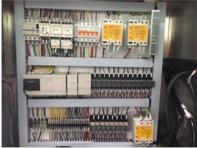
Control Box Mitsubishi, Schneider, CKD, Omron
